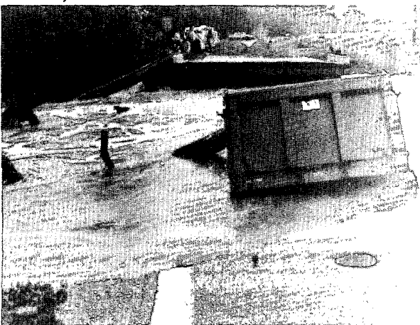
Flooding of Black Creek near Pageland, SC washed out this Highway 43 bridge October 11th. The sand truck above crashed into the creek and was almost completely submerged. Photo courtesy: Photographer-Brian Hough, The Pageland (SC) Progressive Journal.
