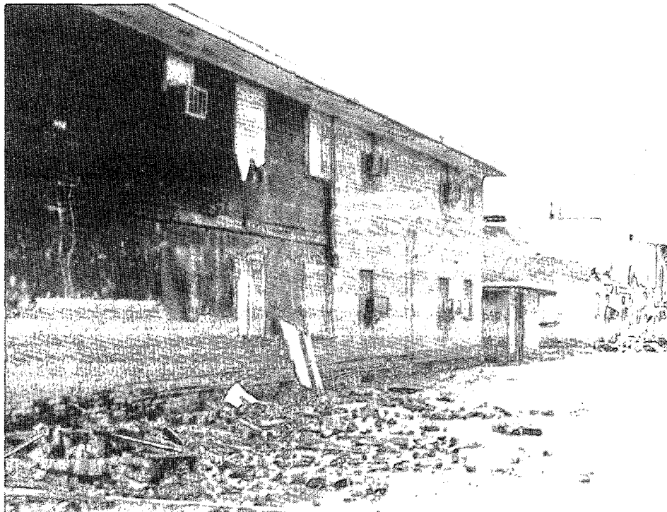
Photograph 5. Damage to two-story brick veneer wall after the Mesquite, Texas tornado. There were no brick ties to anchor the wall to the wooden frame. The wall toppled on the leeward or "suction" side.
