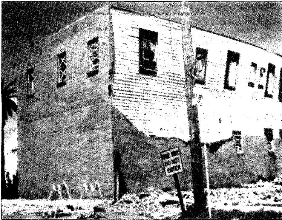
Photograph 6. The same type of damage was found to brick veneer after Hurricane Elena at Gulfport MS. Building response was the same as above regardless whether the wind is from a tornado or hurricane.
