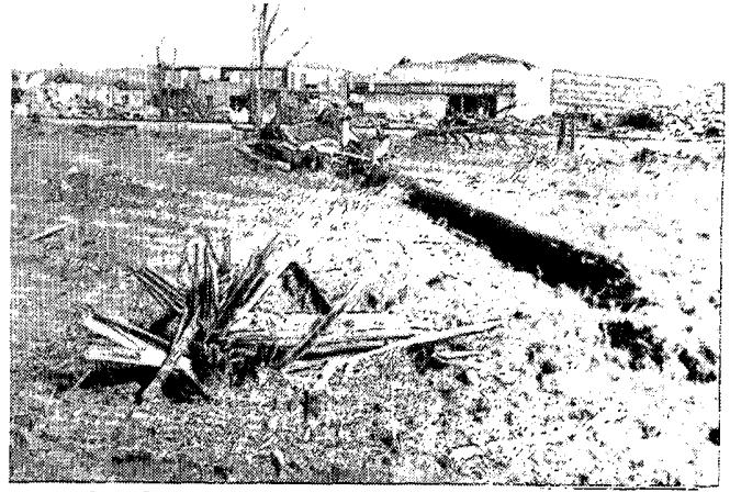
One pole of a two-pole power line structure that was twisted off by the tornado, leaving its stub in an array of splinters.
