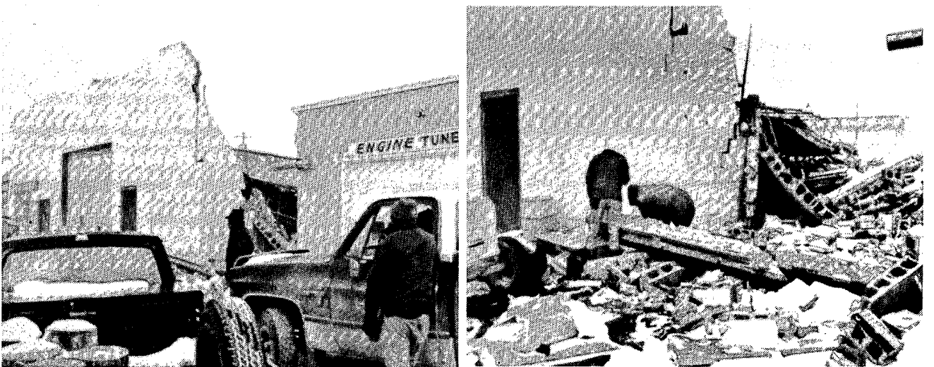
Above are three views of the Hi-Line Masonry building in Shelby which collapsed in on itself during the strong winds on the 30th. According to witnesses, only a portion of the roof was blown off initially, then the remainder of the roof blew upward and the walls caved in a short while later.
