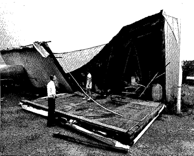
The Ace Service Center manager, left, was inside this 40 x 80 foot, company garage when it partially collapsed during the microburst. The garage, located on Highway 30, lies just out of frame to the right of the Ace sign on the right side of the traffic photo above.
