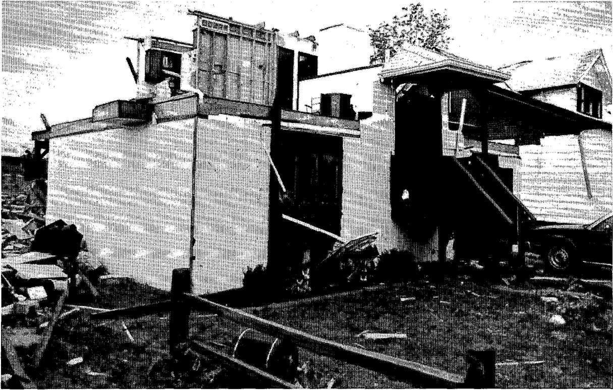
The home on Avenue K that lies just east of the two homes that were blown completely off their foundations. In this case, most of the second floor was removed, but the first floor remained intact and connected to its foundation. ---(SG)
