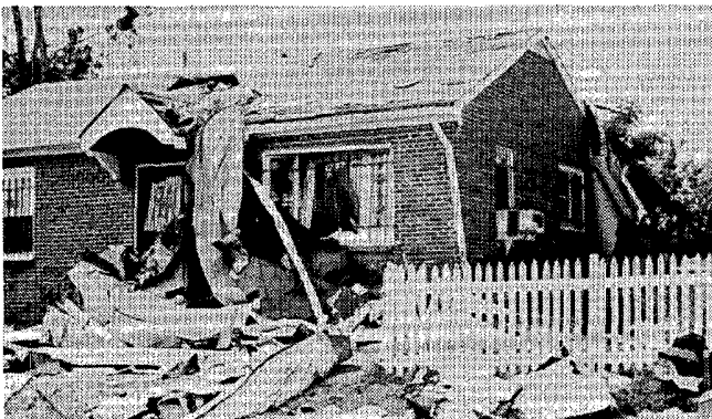
Windblown debris litters a house and yard in east Richmond. The debris is roofing material that came from the nearby Fairfield Elementary School.
