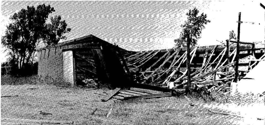
A machine shed at the Mehus farm east of Pickert, southeast of Finley, that was also destroyed by a tornado.
