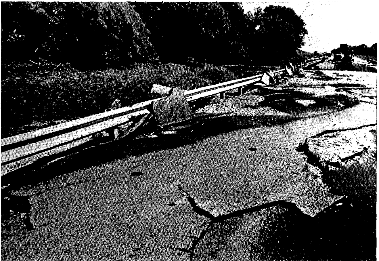
Eight miles south of Comanche, this low section of Texas Highway 16 had large sections of the pavement lifted and carried off the roadbed by floodwaters of Mercer Creek. It was 7 miles upstream of this location that an earthen dam on Lake Eanes gave way, however a second dam on Lake Comanche, about 4 miles upstream, held. Both views above are toward the south, and the direction of flow was from right to left (east).
