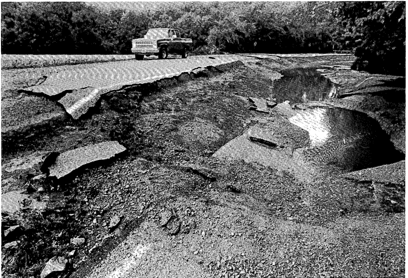
Erosion damage on Douglas County Route 1 near Lone Star.
