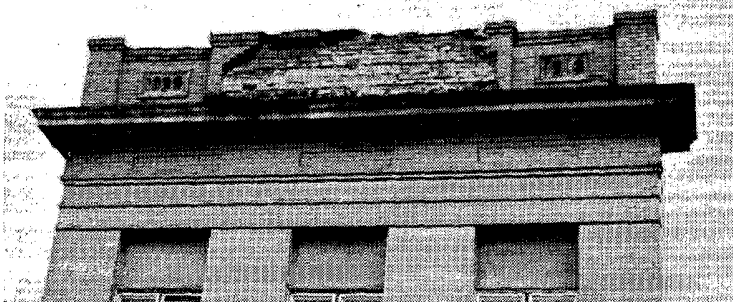
The top of the Norgaard Farm Service building in Finley, from which numerous bricks were blasted out by a lightning strike.
