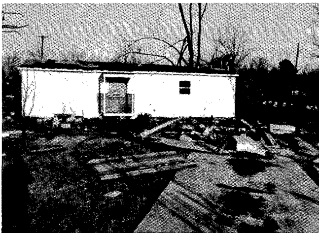
4. Here, an unanchored home at the periphery of the tornado was rotated about the bathroom plumbing.
