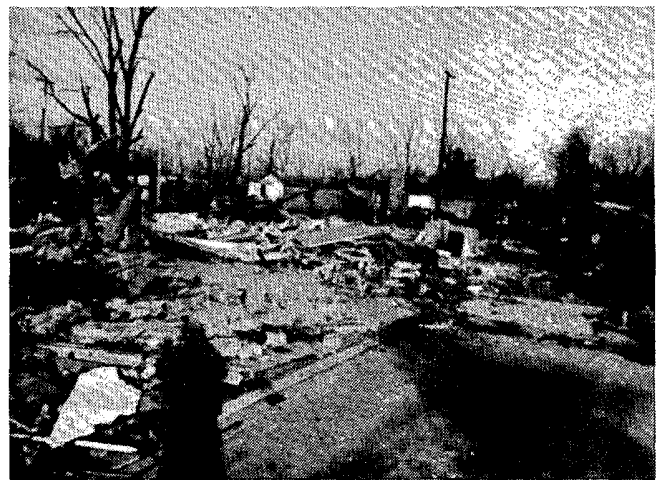
3. A foundation and trail of debris are all that remains of this wood-frame house which, being unanchored, was easily swept away by the tornado.
