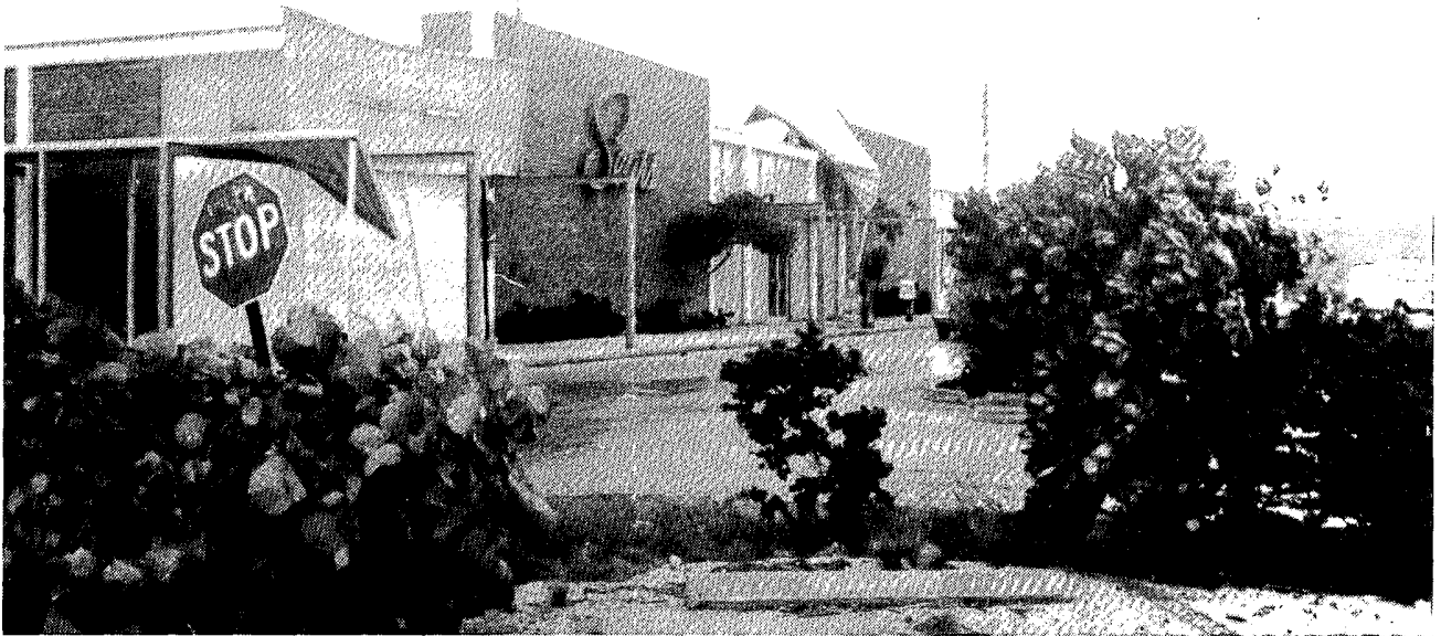
Remains of a sidewalk canopy at a Key West department store after being partially dismantled by FLOYD's winds.
