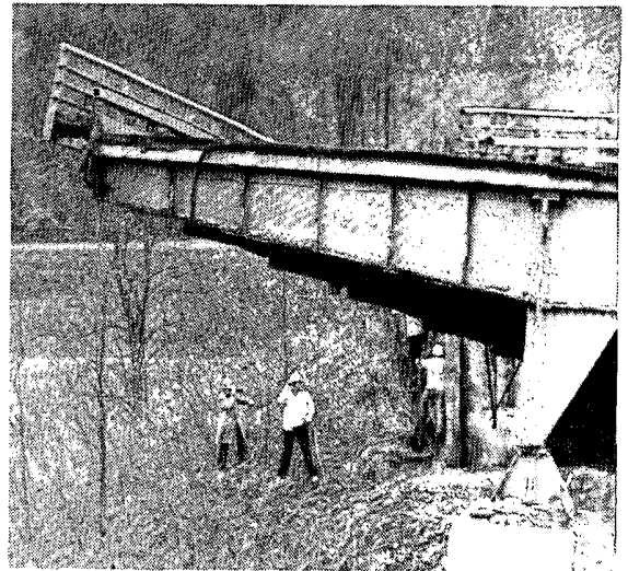
Engineers and officials survey the disaster site to determine the cause of the collapse. The bridge was last repaired 5 years ago and passed inspection only one year prior to its failure.
