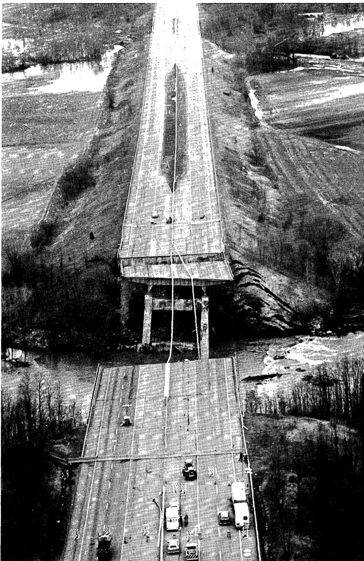
An aerial view toward the west of the gap in the New York State Thruway left by the collapse of the 31-year-old, 540-foot-long bridge over Schoharie Creek west of Amsterdam. ---Photo by and courtesy of The Recorder, Amsterdam, NY.
