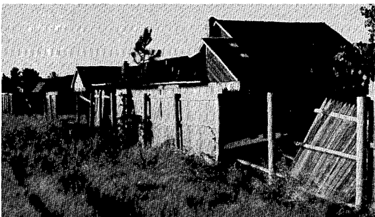
Fence damage caused by west or west-southwest winds on the western edge of the Whippoorwill subdivision (location D, looking northeast).
