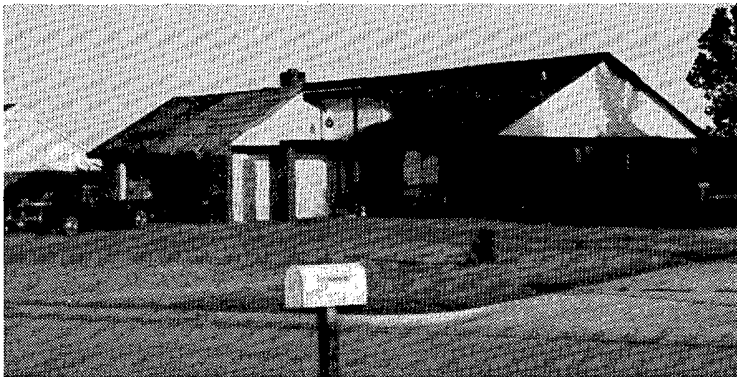
A home in the Whippoorwill subdivision that had a portion of its roof torn off of the front porch and garage (location D, looking south-east). The garage roof was already covered with temporary, protective plastic at the time of the photo.
