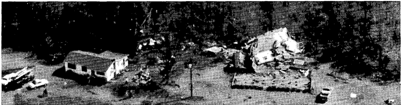
A home that was pushed off its concrete block foundation and subsequently flattened.
