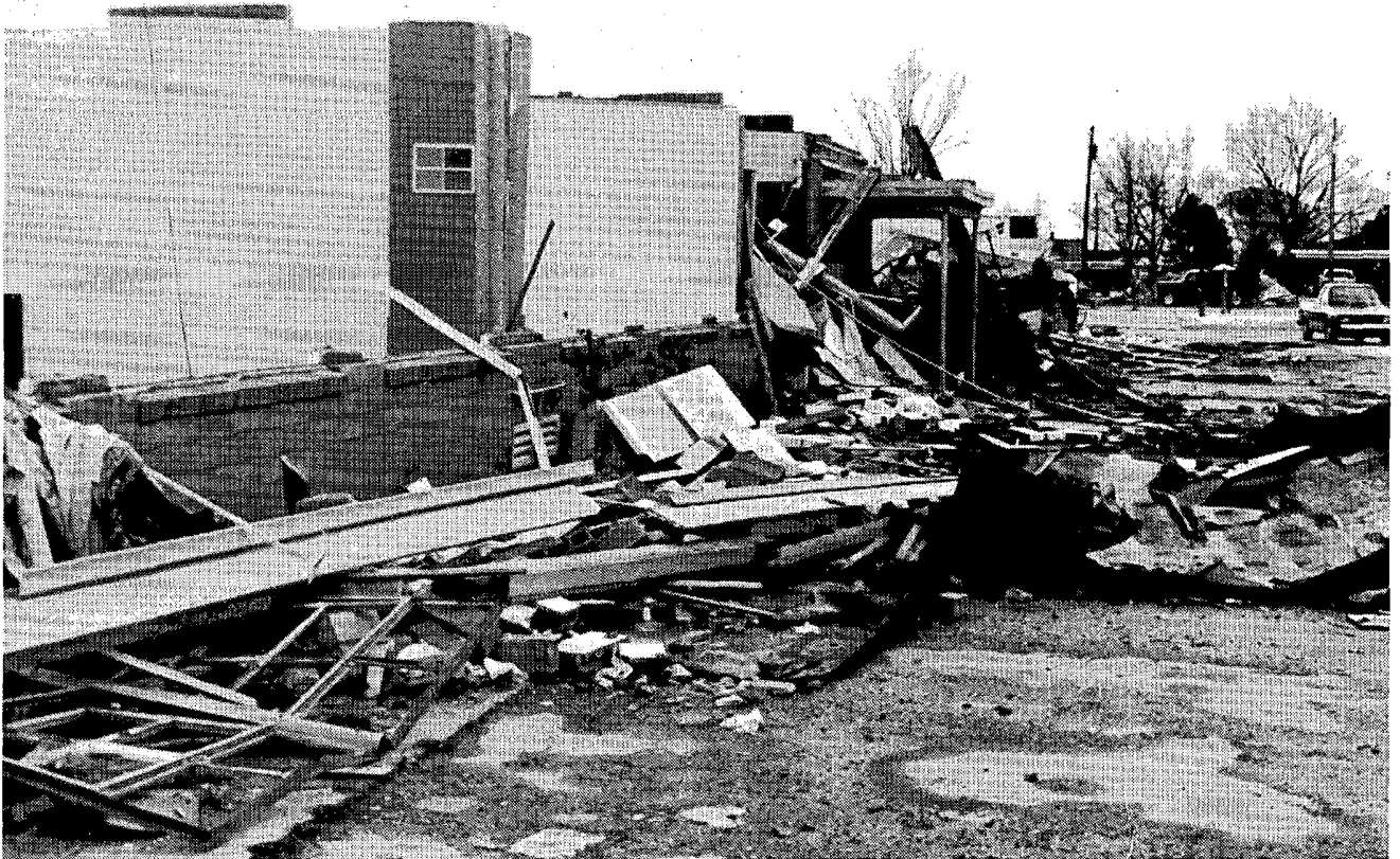
Damage to the junior high school at Wynn where the north wing was unroofed and 2 people were injured. ---All above photos by Allen Lee, NWSFO Little Rock, Arkansas.
