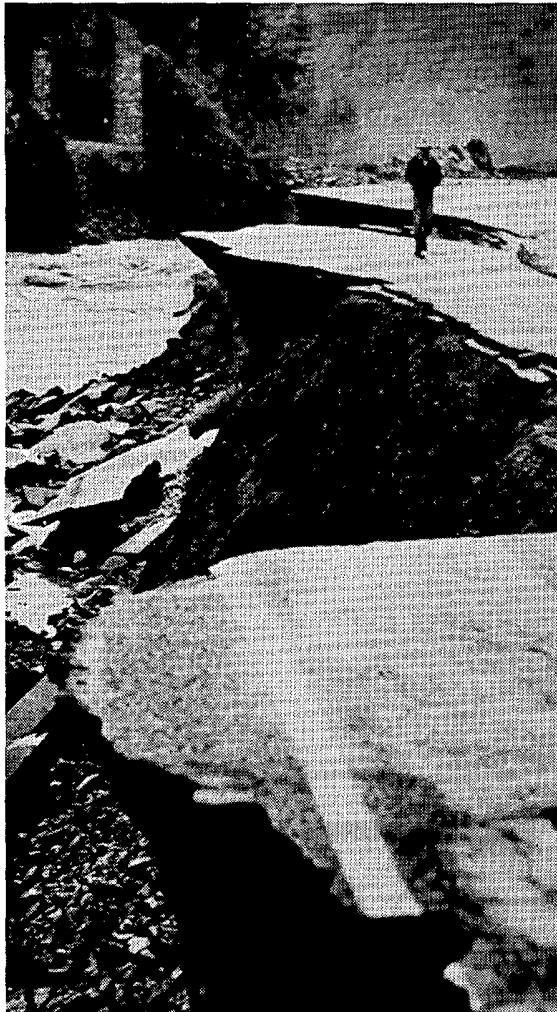
A section of Highway 162 near Covelo, CA, washed out by flooding of the Eel River on February 17th and 18th. ---Phil Toy (via AP).
