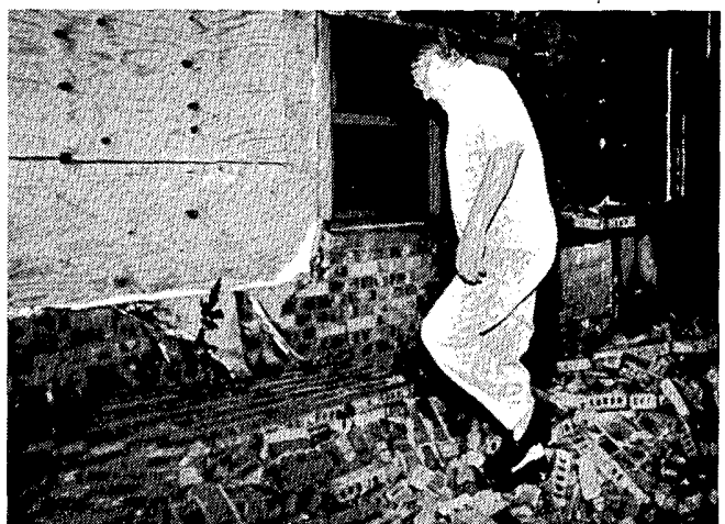
RIGHT: Brick facing peeled from a home by the F3 tornado southeast of Tomball. ---Manuel Chavez, The Houston Post.
