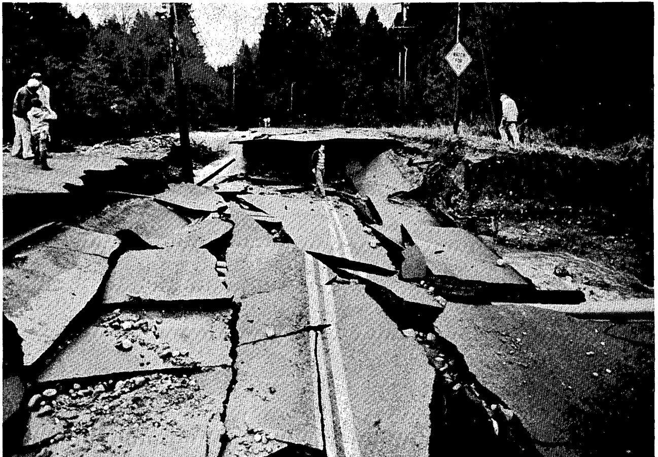
Erosional effects of stream flooding during the storm are well exemplified by this collapsed and fractured road surface. ---(CP)
