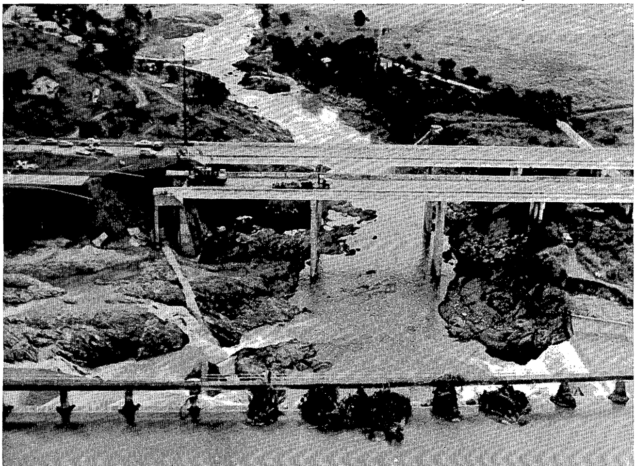
A bridge of the San Juan-Ponce Highway over the Coamo River where pavement leading to it had been eroded away by floodwater which had overtopped the dam in the foreground. A number of motorists had driven into the flooded gap and were washed downstream before anyone was aware of the incident and the road could be blocked off. 29 lives were lost. ---Photo by Victor M. Hernandez, Departamento Recursos Naturales.
