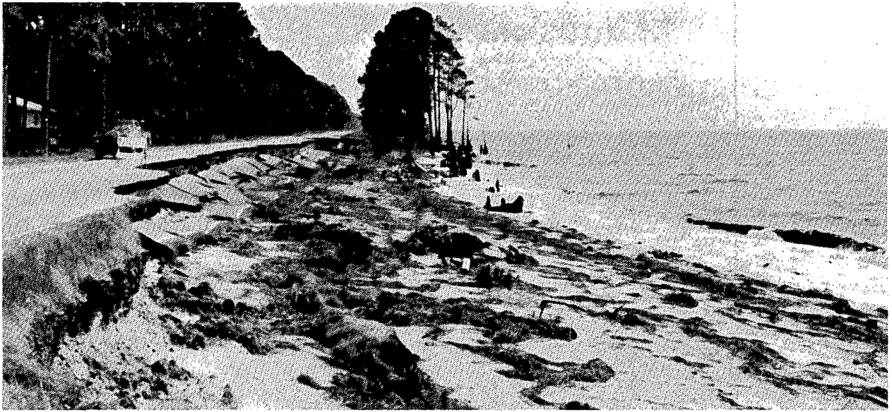
Surge damage to U.S. 98 near East Point, approximately 10 miles east of Apalachicola, Florida.
