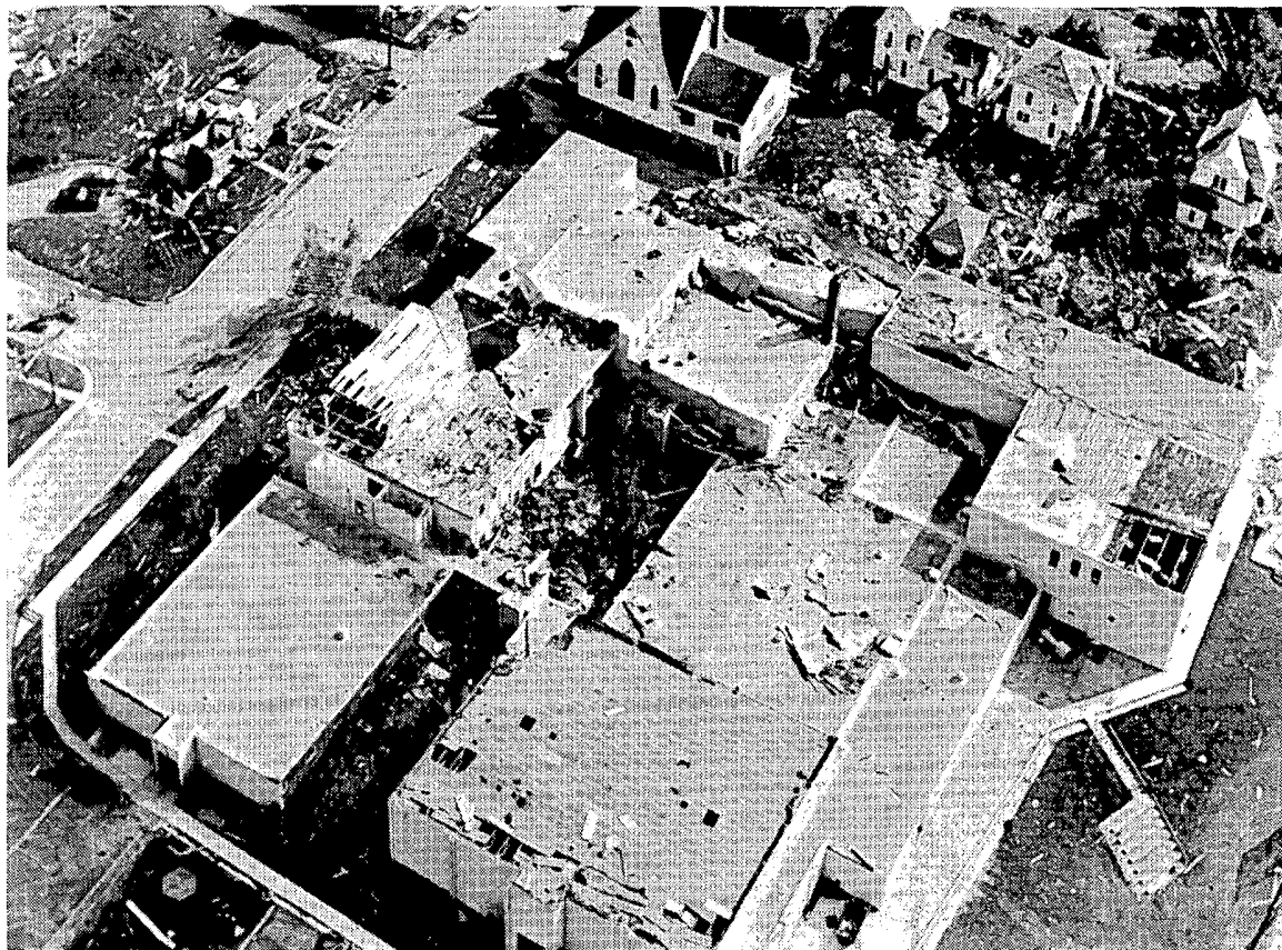
Roof damage to the Barneveld High School. An impression was left in a gymnasium wall after it was struck by a flying auto. (CT)
