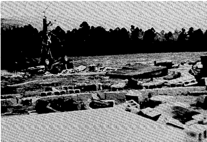
A ground view from the foundation of the home in the top photo.
