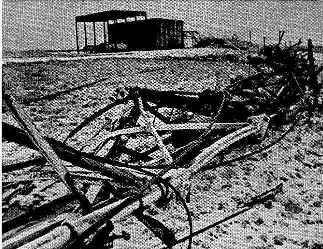
Twisted skeleton of the 1439 foot tower of KLDH-TV of Topeka, KS. The tower buckled and collapsed under the weight of a 3 inch thick coating of ice. ---Photo by Kathy Borchers, Topeka Capital-Journal.
