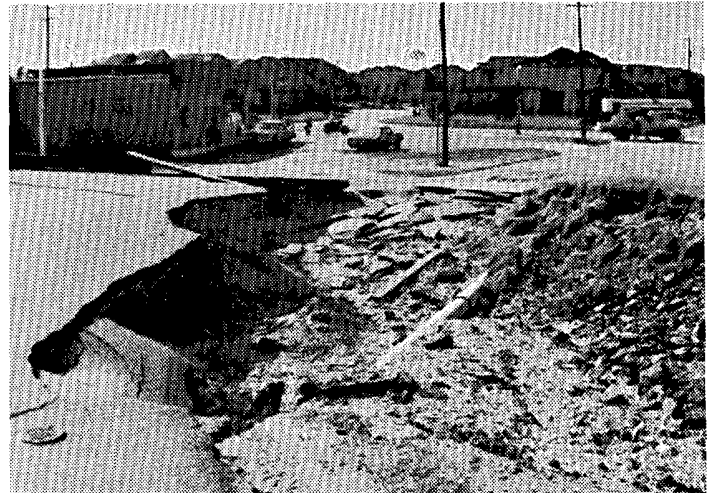
Storm surge erosion of a roadway on the inland side of Seawall Boulevard in Galveston.
