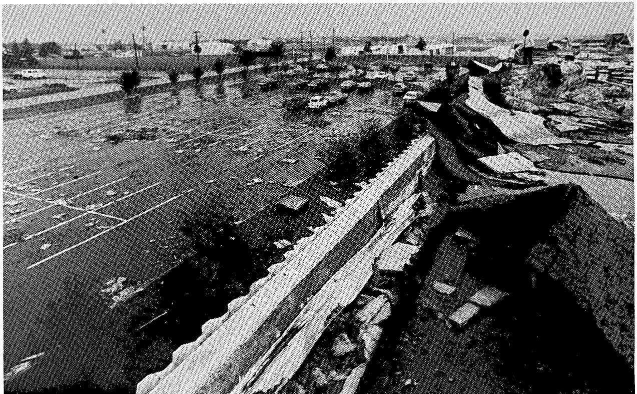
Debris from the damaged roof of a manufacturing plant litters the adjacent parking lot. The location is an industrial park near the A-B-E Airport. ---Photo by Jim Battles, The Allentown Morning Call.
