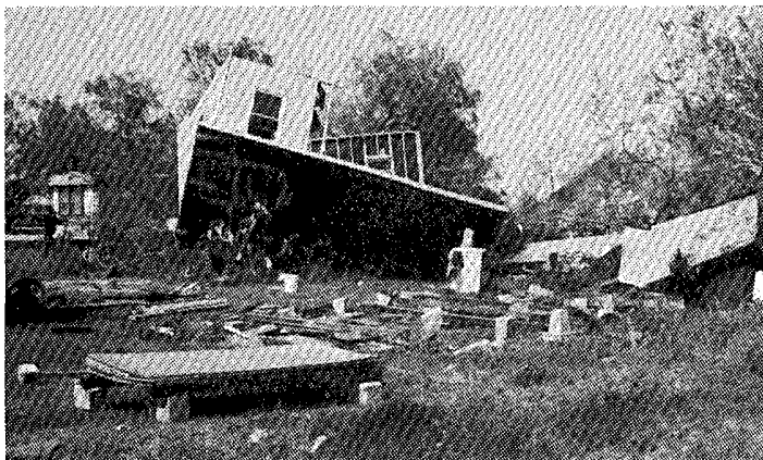
Overturned house which originally sat on the concrete pillars in the foreground.
