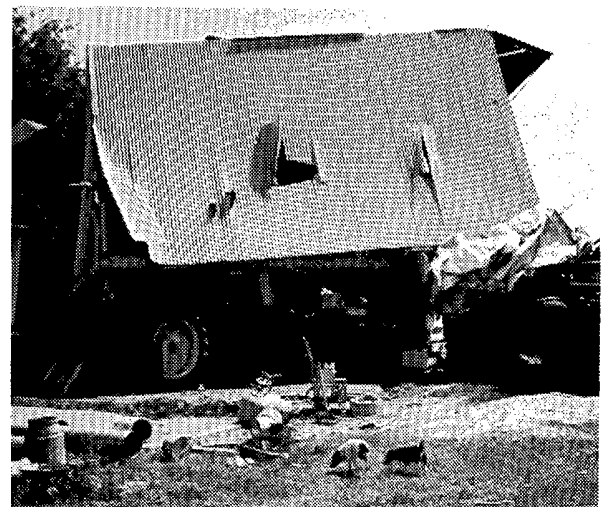
Machinery shed in which concrete foundation was pulled out of ground.
