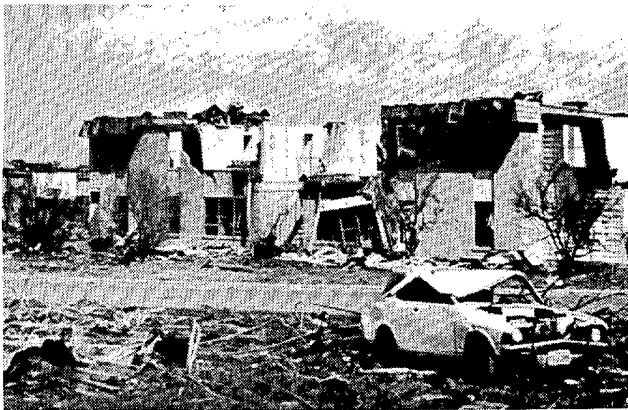
An apartment building and auto struck by the Paris Tornado.
