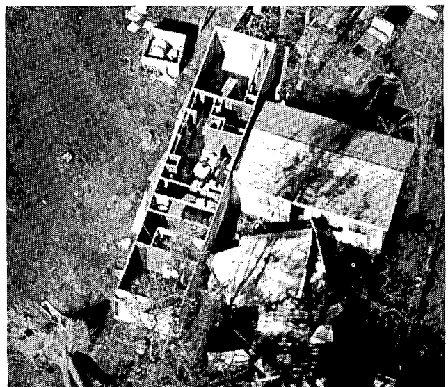
The roof peeled from a trailer attached to a house southeast of Hope, Arkansas. (HS Photo)
