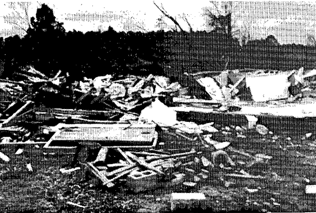
A frame house carried from its foundation site, 4.5 miles southwest of Nashville, Ark. A woman inside, carried about 200 ft., received only minor bruises. (NWS Photo)
