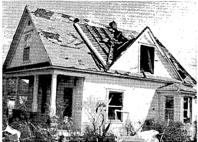
A house with roof damage in Mulberry, Ks. ---Photo by Max Griffith, NWS Wichita, Ks.
