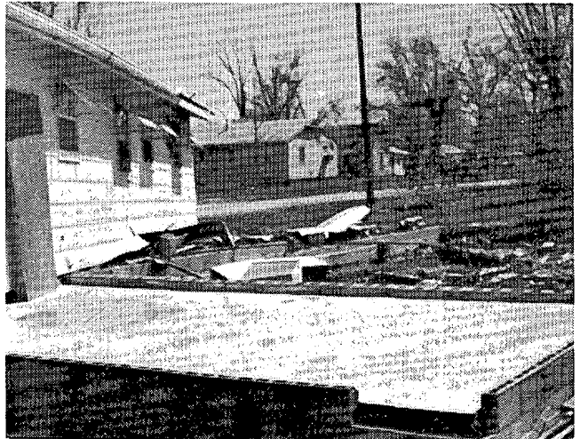
A house rotated 30° off its foundation. ---Photos supplied by NWSFO St. Louis, Mo.
