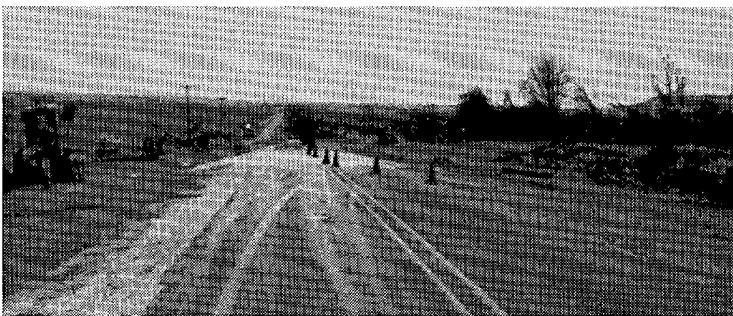
25 feet of pavement peeled off of Texas Highway 382 by the tornado's winds.
