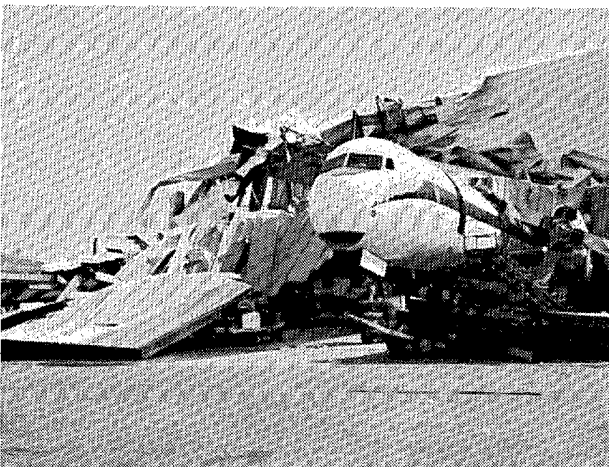
Aerial view (top) of the damaged hangar housing the Zantop Airlines Maintenance shop (looking south). Damaged hangar and aircraft (looking east).
