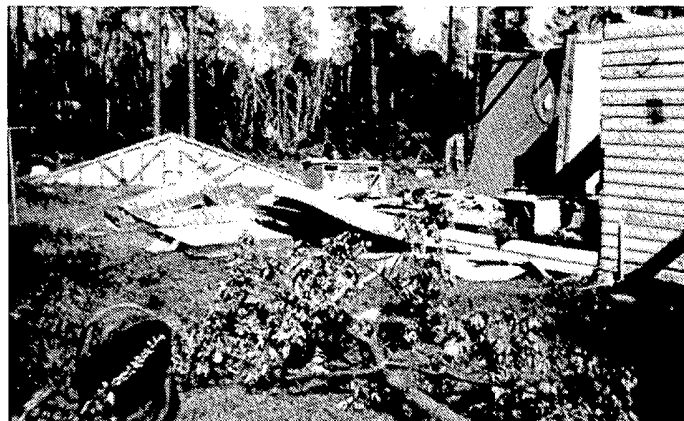
B. Roof and rear walls torn off
