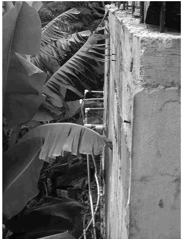
Photograph by: Bill Rohring, DPNR-CZM Irrigation from stormwater cistern
