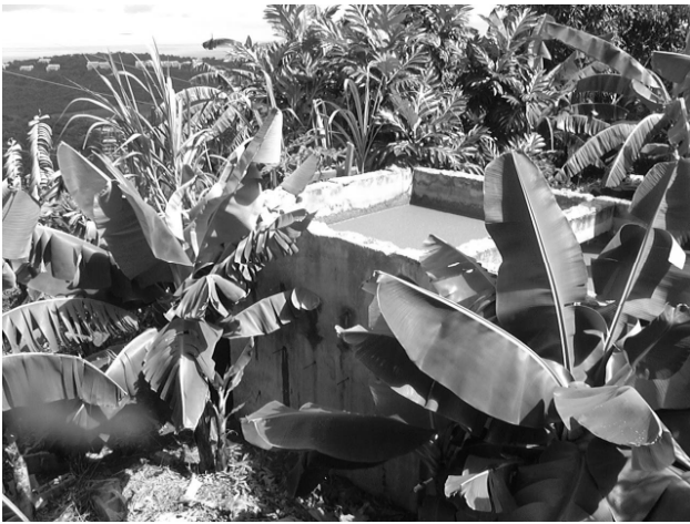
Photograph by: Bill Rohring, DPNR-CZM Stormwater Cistern
