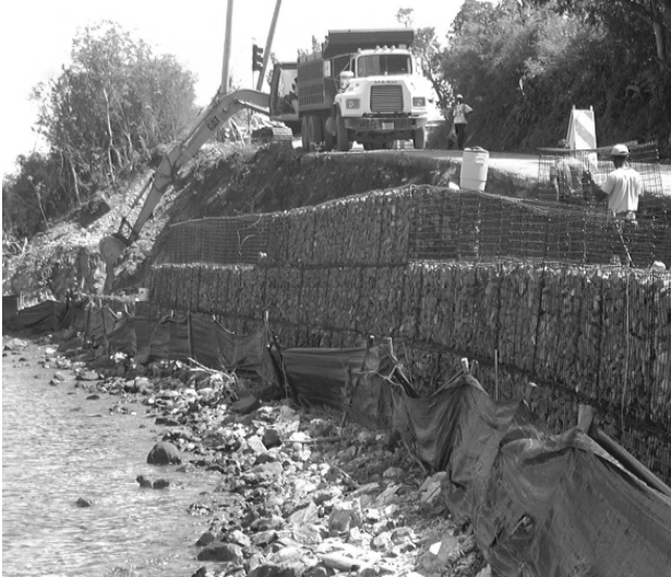
Photograph by: Bill Rohring, DPNR-CZM
