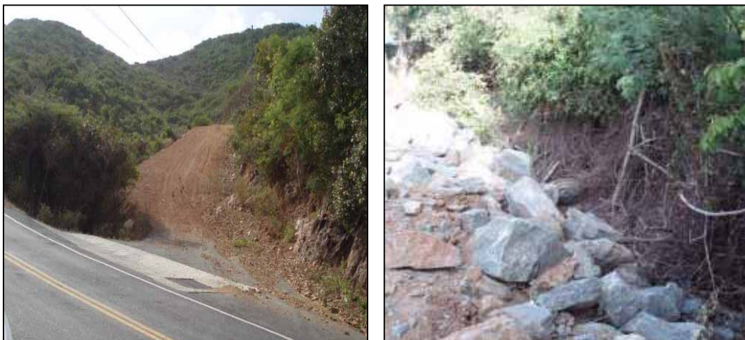
Figure 6. Drainage "improvement" below dirt estate road in Johns Folly Bay (left), creating severe gut erosion behind private residence. DPW temporary fix with rubble/rip rap (right).
