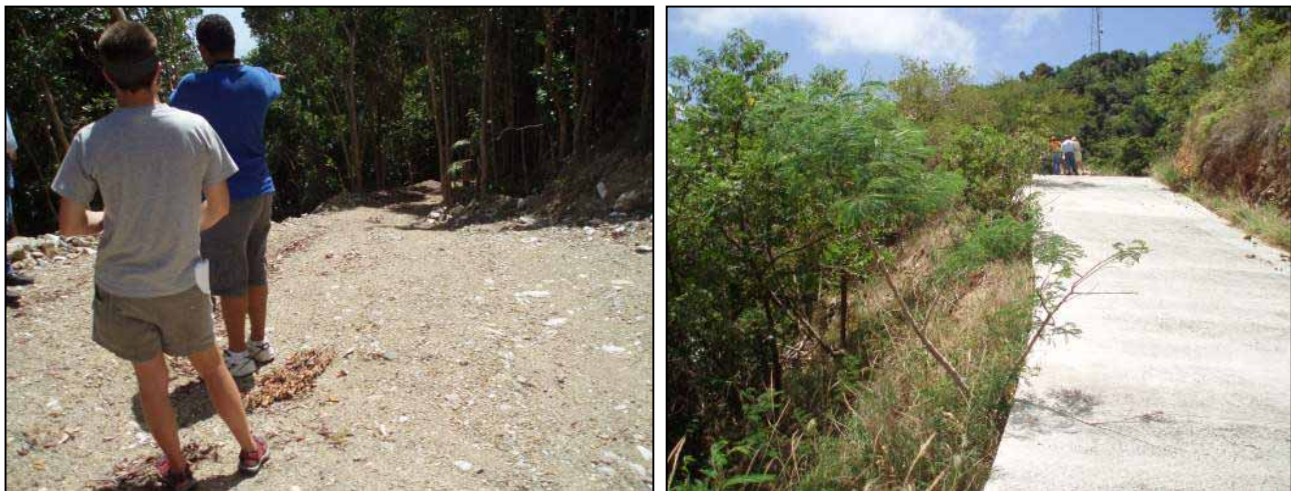
Figure 9. Two locations where field team observed road cutting/filling (left) and paving (right) conducted without appropriate permitting.
