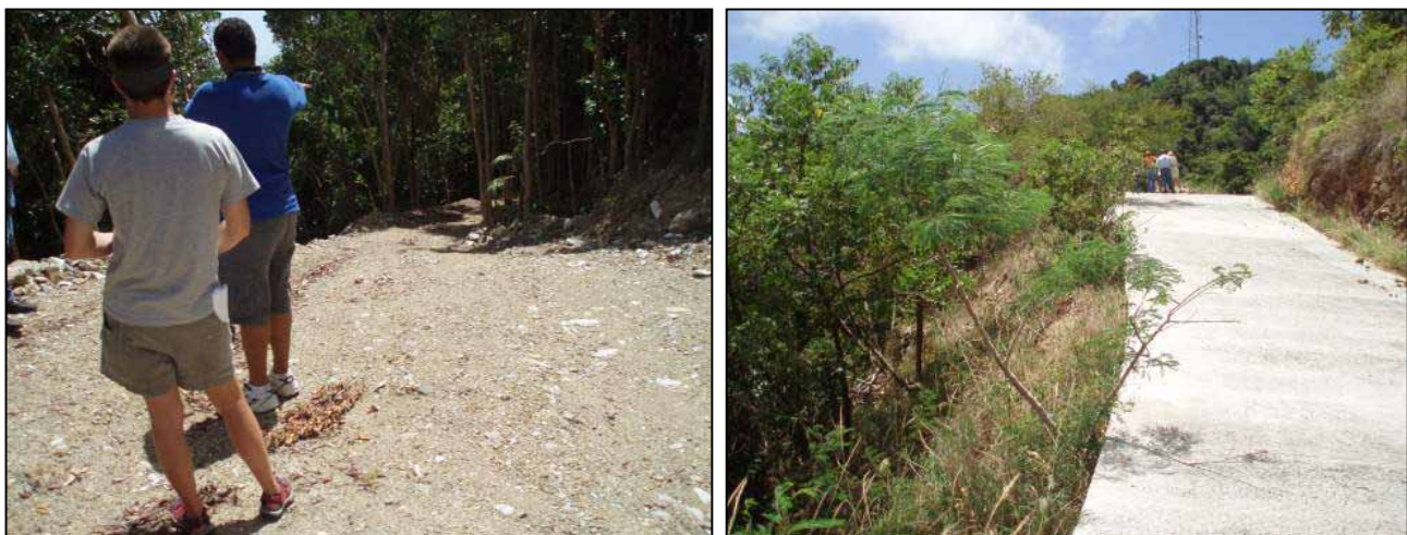
Figure 9. Two locations where field team observed road cutting/filling (left) and paving (right) conducted without appropriate permitting.
