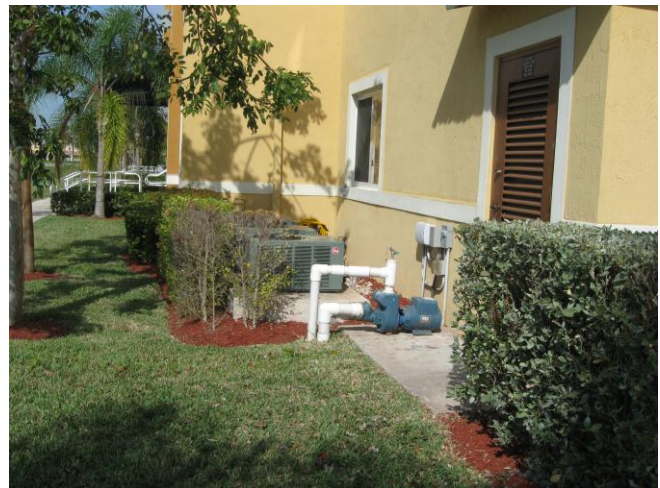
Figure 13. This pump draws water from the stormwater pond in Figure 14, and this water is used for site irrigation. Photo Source: CWP.
