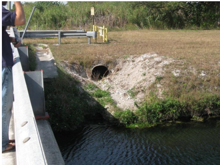
Figure 15. Canal maintenance is completed by the local government or the SFWMD. Photo Source: CWP.
