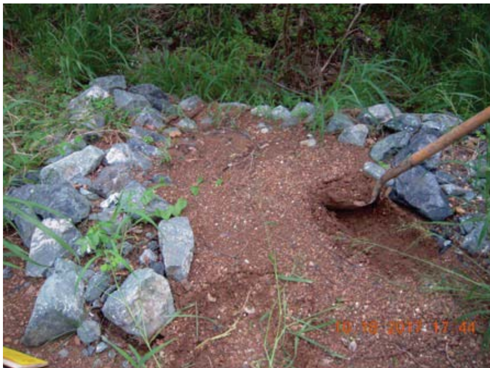
Figure 35: Damaged sediment trap
