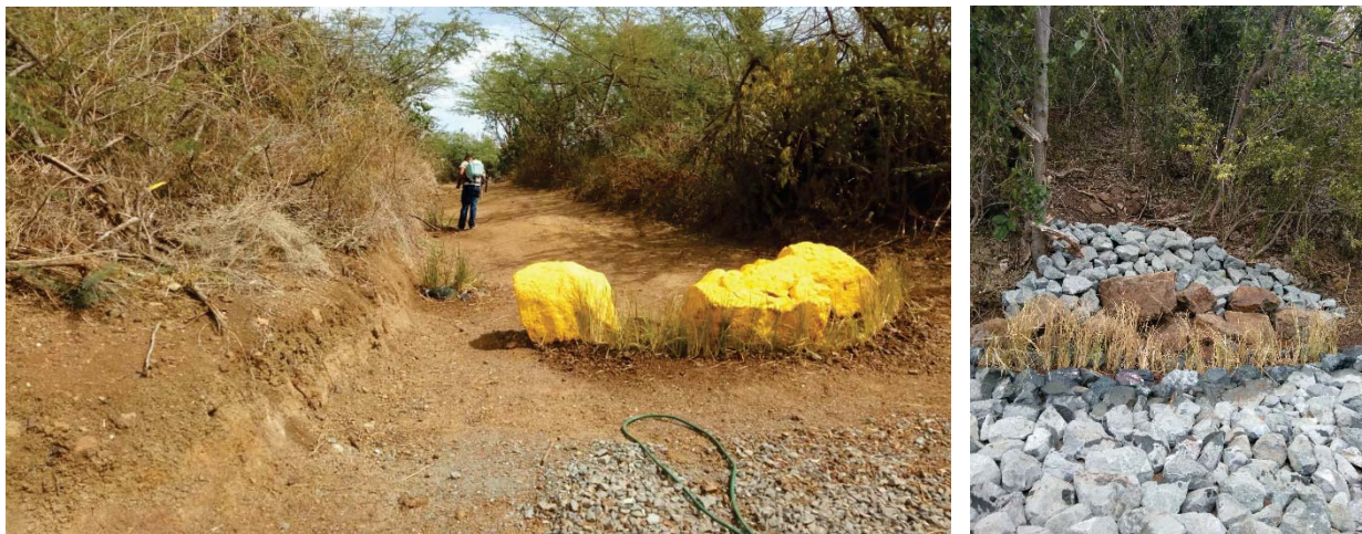
Figure 17. Some of the practices implemented on the closed segment of the road.
