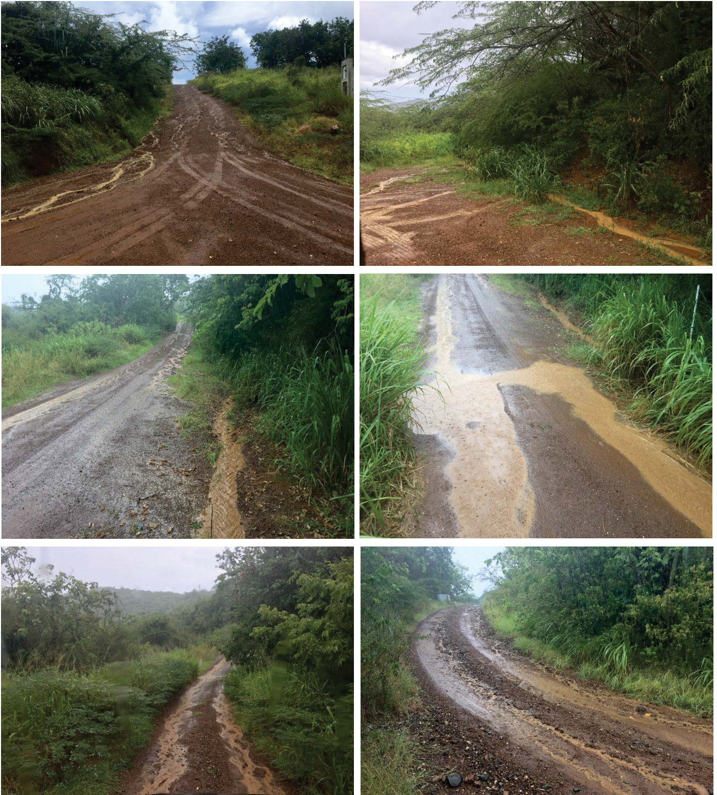
Figures 2. Sediment runoff and accumulation along dirt road at Punta del Viento during a small rain event prior to stabilization.
