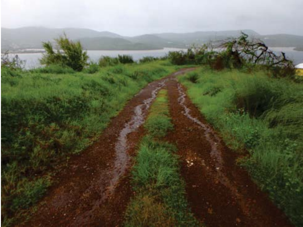
Figure 32: Runoff flowing through the center of the road and not being delivered to the ditch on the right were the sediment traps are located
