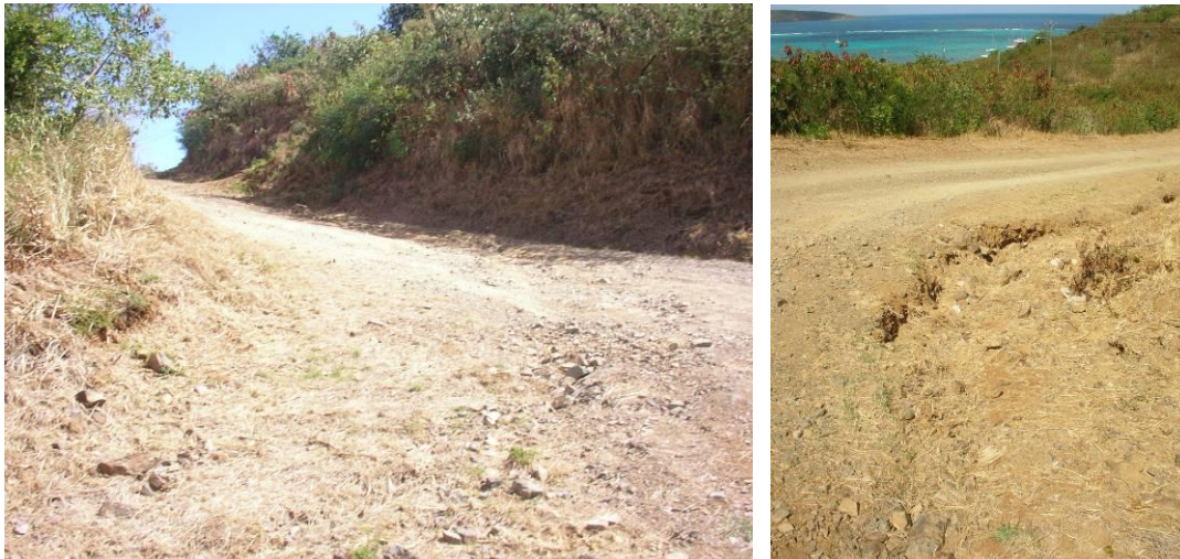
Figure 5.7. Gullying and erosion observed along Ridge Rd.
