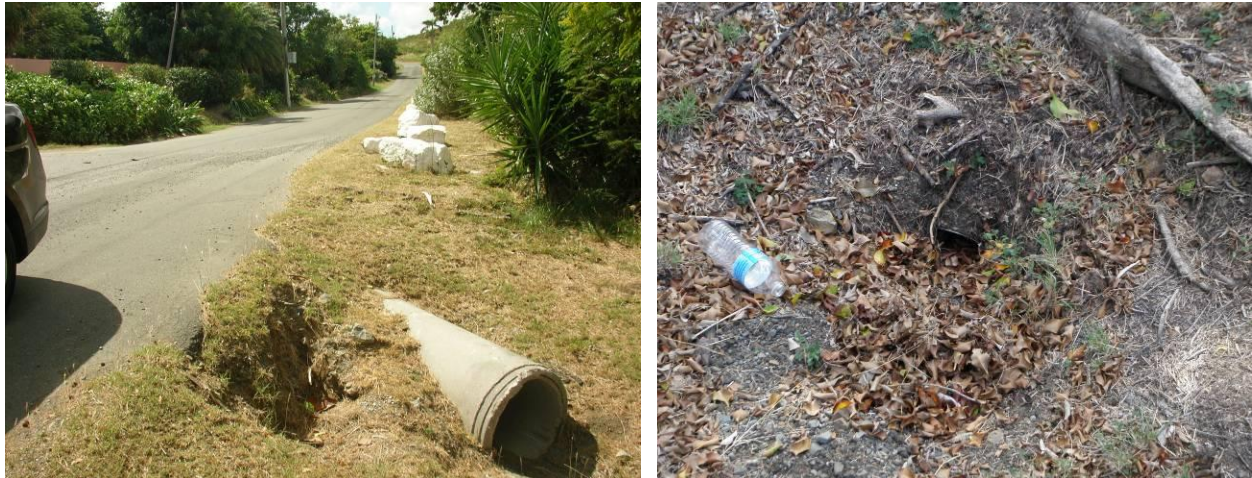
Figure 3.14. Examples of collapse at road edge in the Punnett Bay area (left), and a completely clogged culvert in Southgate Farm/Anna’s Hope (right).
