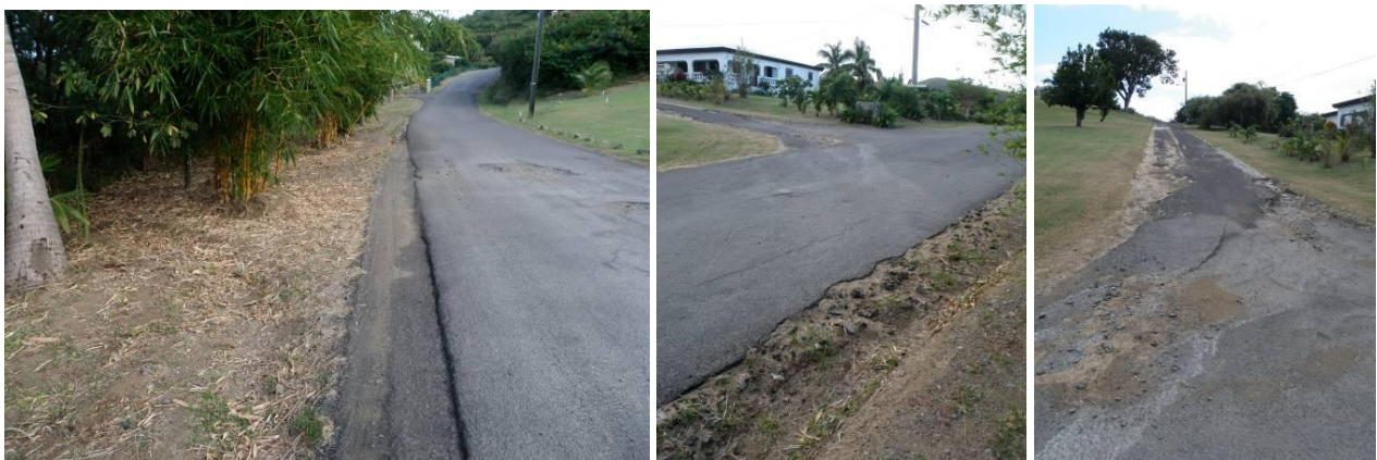
Figure 3.7. Road drainage from residential areas leading to gut erosion.
